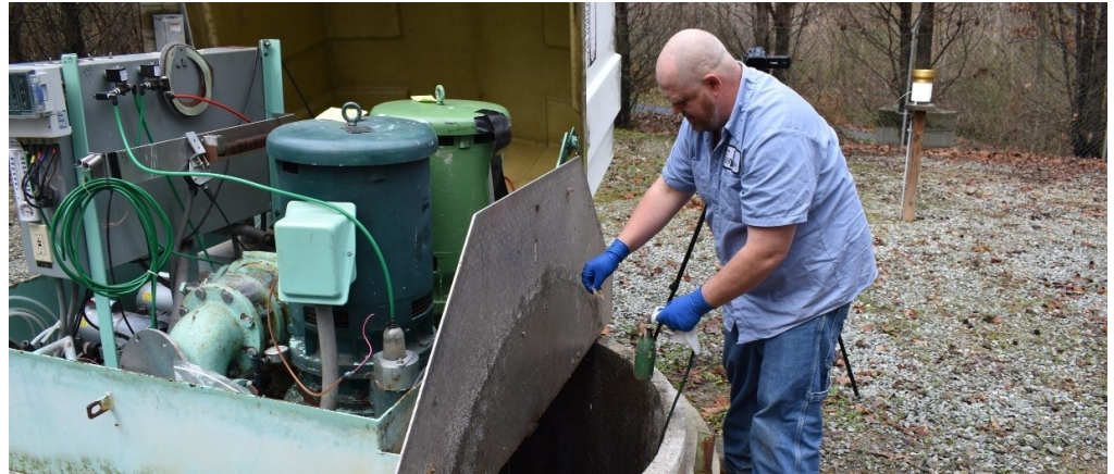
COLLECTION TEAM: Wastewater collection employees are highly certified and continually evaluate and maintain the town's system of sewer manholes, pipes, and pump stations to ensure the system is operating properly and to prevent spills. See Water Distribution and Wastewater Collection page.
