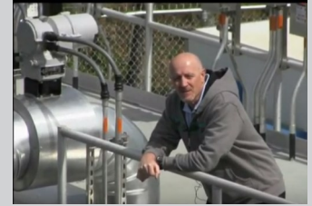
Deputy Utilities Director—Water Treatment Jeff Mahagan leads tours of the plant. See a video on how wastewater is treated and returned to the Eno River in Hillsborough (available on the town’s website and YouTube
