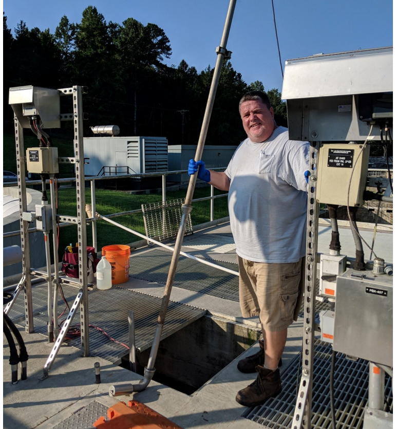
Chief Wastewater Plant Operator Shawn Maines performs monthly maintenance on a turbidity and suspended solids probe, one of 12 probes for various measurements at the plant. He started as a wastewater plant operator I for the town in 1998 and earned operator II and III titles over the years, with the operator III designation signifying he has obtained the highest level of certification in wastewater treatment.
