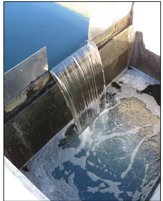
The Wastewater Treatment Plant takes dirty wastewater and turns it into crystal clear, clean water before returning it to the Eno River.
