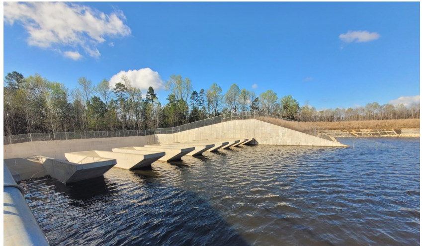
The reservoir's new spillway is designed with notched weirs, also called piano keys because they resemble the instrument's keys.
