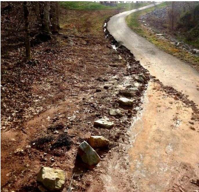
Erosion and sedimentation from stormwater runoff may be considered unreasonable use depending on the individual situation.
