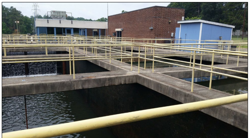
Sedimentation basins at Hillsborough Water Plant
