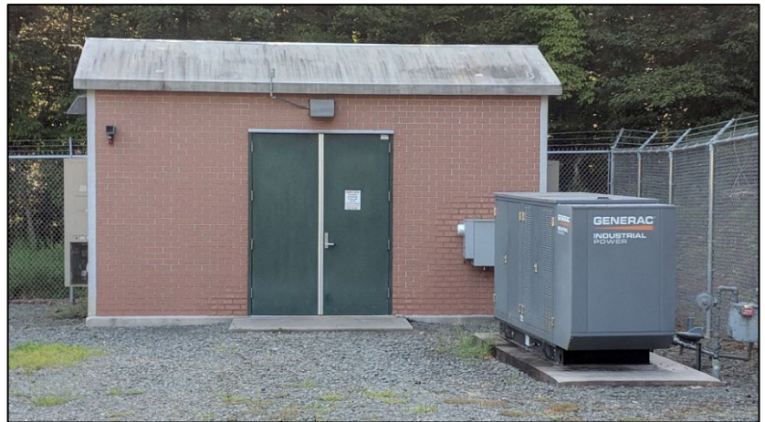
This building houses a pump station on Elizabeth Brady Road. A generator helps ensure it continues to operate, preventing sewer spills.
