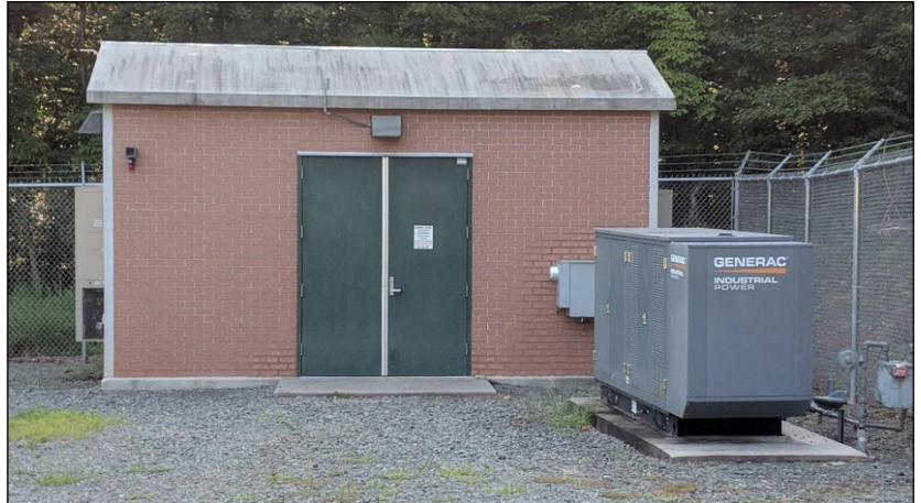
This building houses a pump station on Elizabeth Brady Road. A generator helps ensure it continues to operate, preventing sewer spills.
