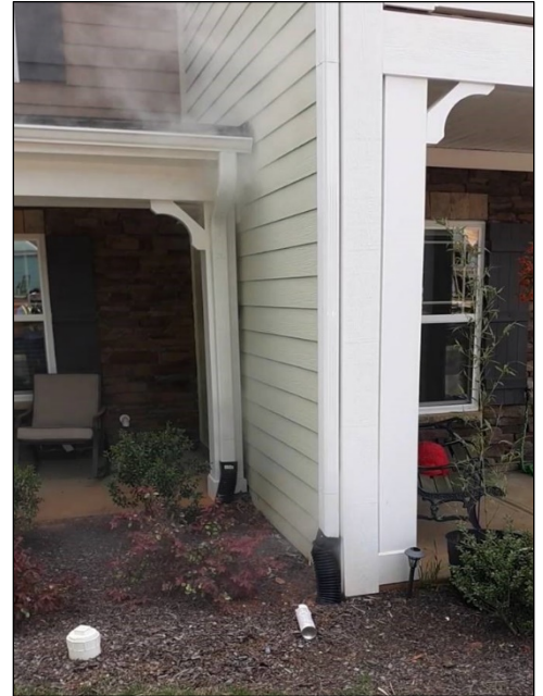
Smoke testing of sewer lines found storm gutters erroneously connected to the town’s sewer system on this house.
