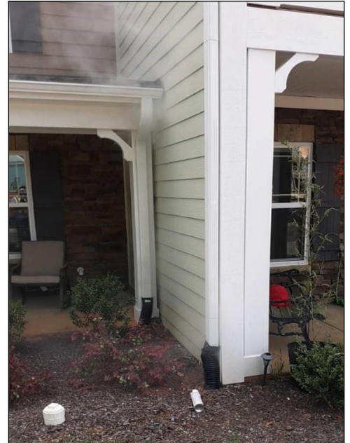
Smoke testing of sewer lines found storm gutters erroneously connected to the town's sewer system on this house.
