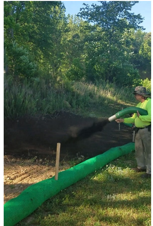
Compost being blown in place for the Cates Creek Park compost blankets.
